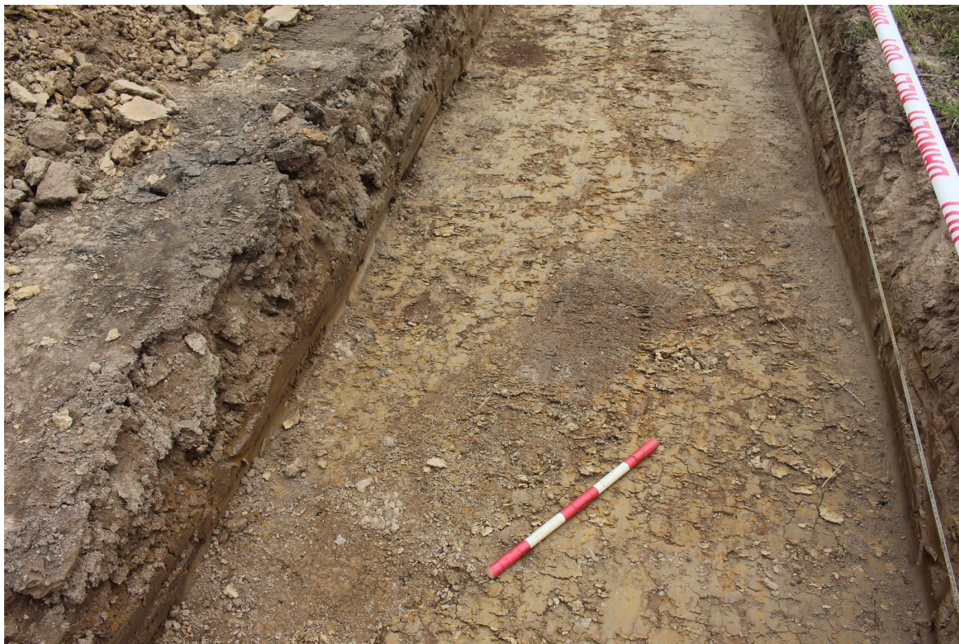
T01 – Service cut on same alignment as previously identified probable water pipes. The date of the pipes is uncertain, but they appear to be established after the tramline has gone out of use.
